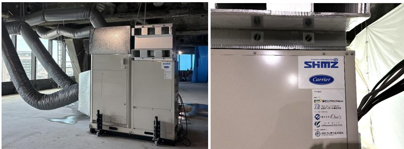
Carrier Japan's Single Ace™ packaged air-cooled air conditioning unit serving as the core of the temporary cooling system deployed at the TOKYO TORCH Torch Tower construction site
